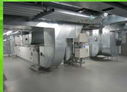
Figure 7: WPE plant (ventilation) hall
