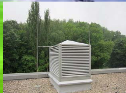
Figure 9: Effluent exhaust at WPE rooftop
